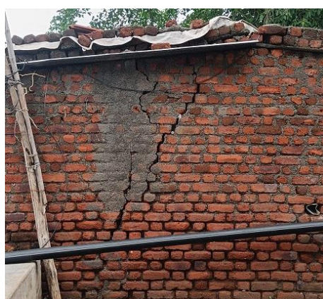
Photo; 3 Visible cracks, crevices, cattle shed and room attached in the home at farm
